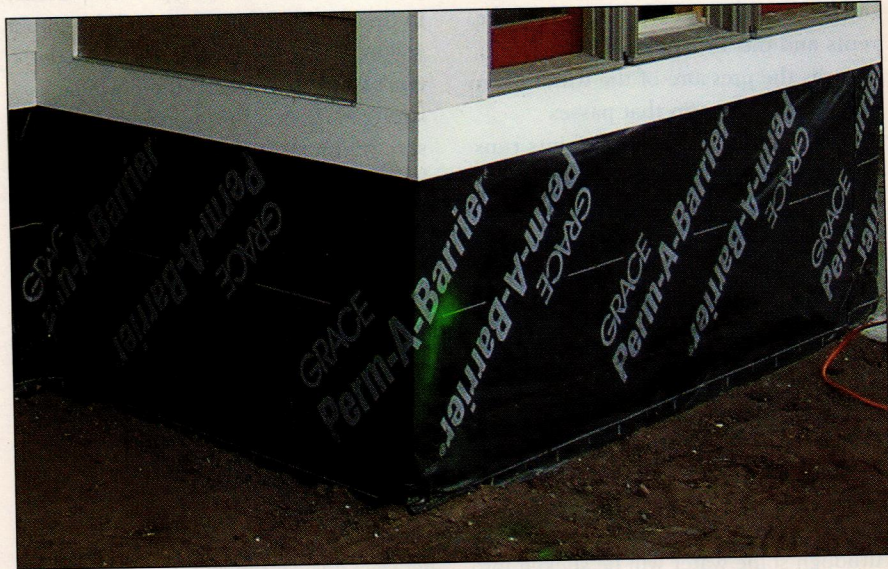
FIGURE 1. The key to wind-smart detailing begins with a continuous air barrier. While ordinary housewrap might work, a self-adhesive membrane applied to continuous sheathing is more durable and less likely to leak once installed. In heating climates especially, it's important to use a specially formulated membrane (or comparable spray-on liquid) that will not create an exterior vapor barrier.
