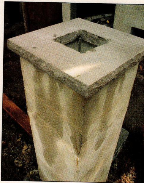
FIGURE 2. Column bases are tied to the foundation grid below grade. Above grade, Saduk's crews lay up 4-foot piers of 16-inch-square concrete masonry block, with fully grouted cores. Capping the block pier is a 20-inch-square bluestone slab, with a 6-inch-square hole in the center to receive the base of a 6x6 treated-wood post. The anchor bolt (top, center) will hold down a galvanized steel engineered standoff post base connector for securely attaching the wood post to the concrete pier. This block pier has already received a stucco scratch coat and will be given additional cementitious finish coats.
