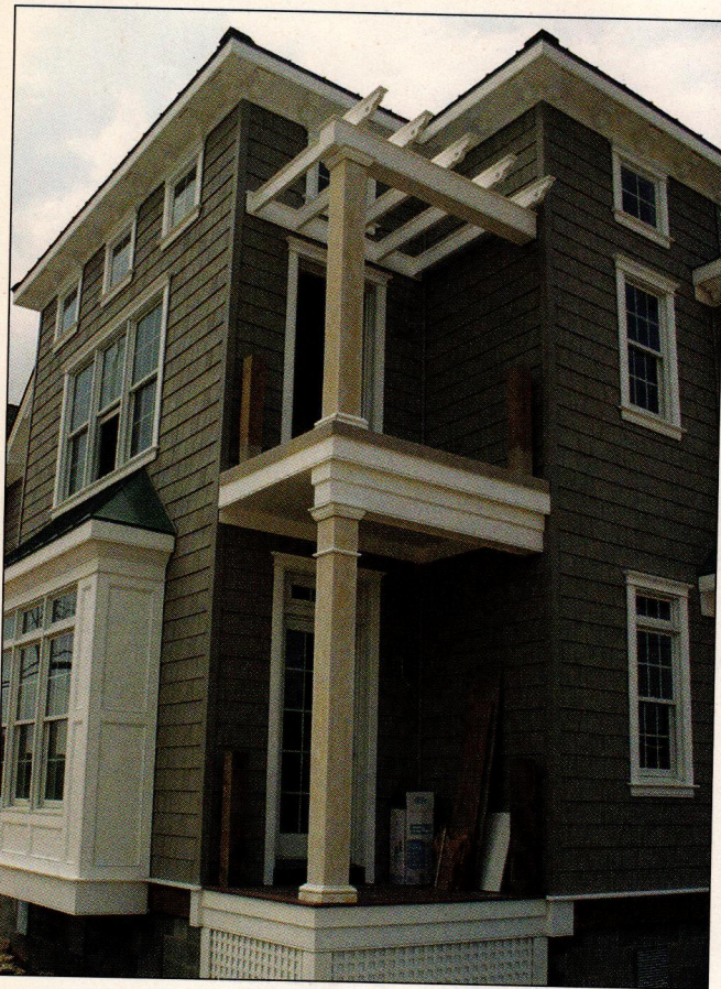
FIGURE 1. The column shown above is designed to carry an upper-story porch; details may vary slightly for columns that carry both an upper deck and a lower deck. However, the principles are the same for any porch/deck configuration, as detailed in the illustration on page 27: The exteriors are composed of layered, weather-tolerant, low-maintenance synthetic materials, while the inner structures are strengthened by reinforced masonry, engineered connectors, and treated wood.
