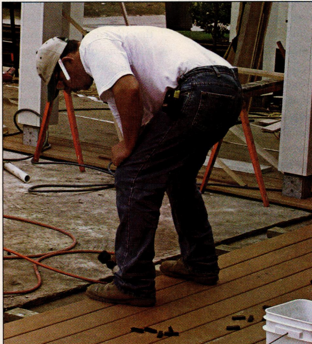
FIGURE 5. Borden relies on hidden deck fasteners when zoning requirements allow. He typically uses Eb-Ty "biscuits" (top left) that get installed in a kerf cut in the edge of a board with a plate joiner, or Tiger Claw fasteners (top right). The Tiger Claw install faster in hardwood, but they're difficult to pound into the edge of composite decking. For composites, it's better to use the decking manufacture's proprietary fasteners, such as those made by Eb-Ty for CorrectDeck (above).
