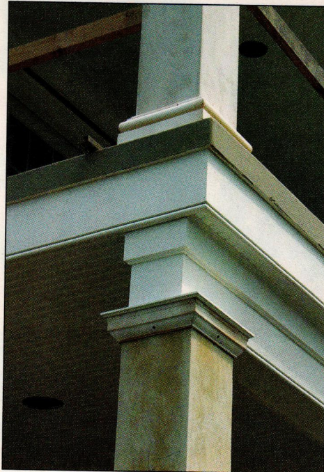
FIGURE 3. The porch's wood and steel structure is completely hidden once the porch receives its layered trim treatment of Azek ceiling beadboard, tooled Azek trim, and Fypon column base and capital moldings. In addition to its decorative purpose, the completed porch is able to shoulder its part of the design wind loads typical for a coastal home.
