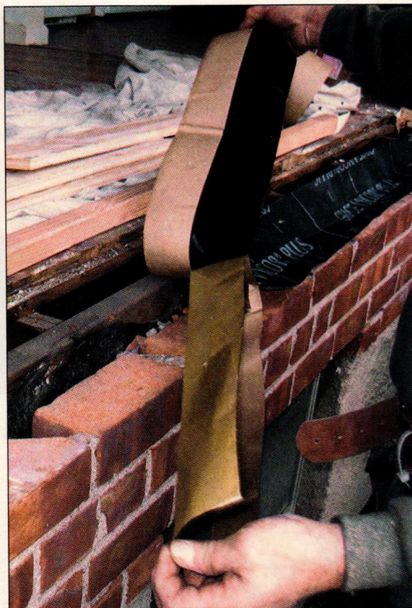
FIGURE 2. Deck-level sliding doors are susceptible to water and air infiltration. To reduce problems, the author begins with a layer of self-adhesive flashing beneath the subfloor and lapped onto the brick veneer.
