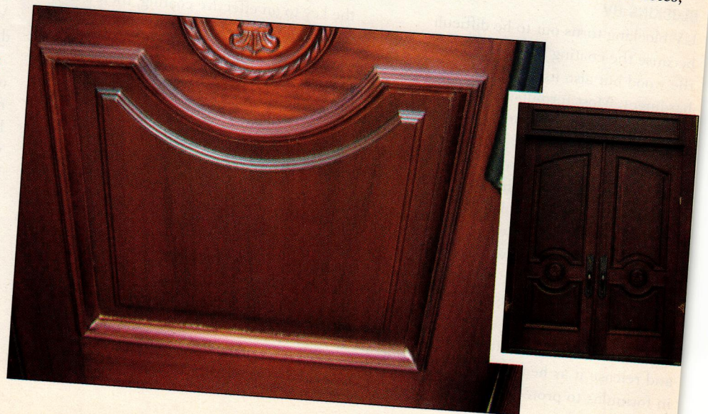
FIGURE 2. At right, two doors on opposite sides of the same street show the effects of different solar exposures. The two-part polyurethane clear coat on a mahogany door on the sunny side of the street (right) is beginning to whiten and crack after just two years in the sun and will soon need to be stripped and reapplied. The same finish on a white oak door on the shady side of the street (far right) is still going strong after five years in place. "Wind and rain don't have that much to do with finish performance," explains finisher Dave Anderson. "It's mainly the sun." However, once the finish begins to fail, water damage to the underlying wood becomes a risk, adding urgency to the need to refinish.
