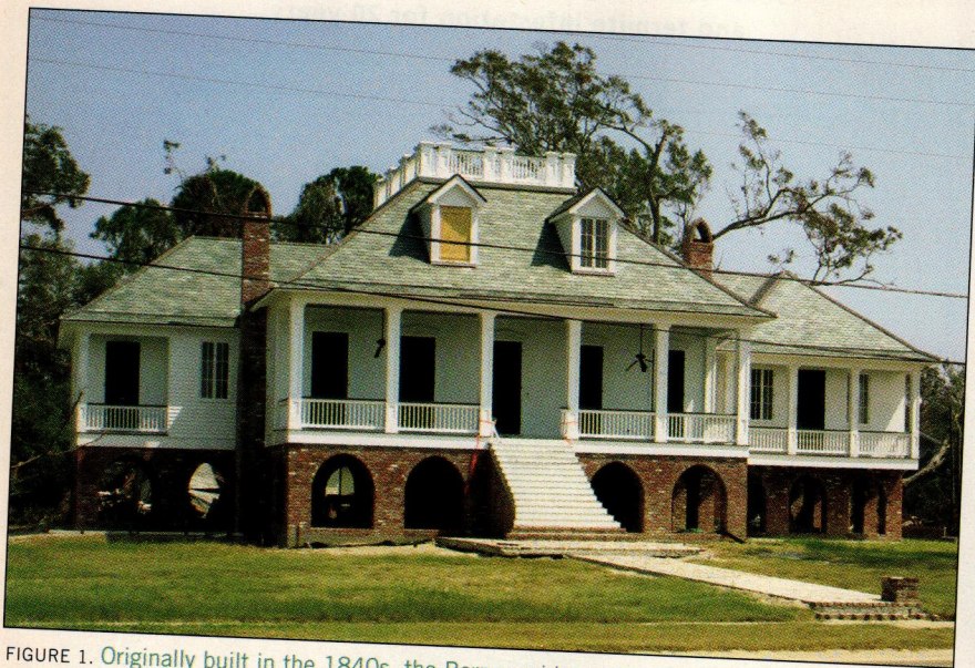
FIGURE 1. Originally built in the 1840s, the Borne residence (above) suffered only minor damage during Hurricane Katrina. Wind damaged an upstairs window, and the surge washed out the stair railings, but otherwise the home stood firm. Unfortunately, homes on either side of it (right, top and bottom) did not fare as well.
