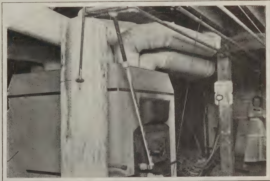
View of "Leader" Furnace in the Cellar, Showing Pipe Connections
