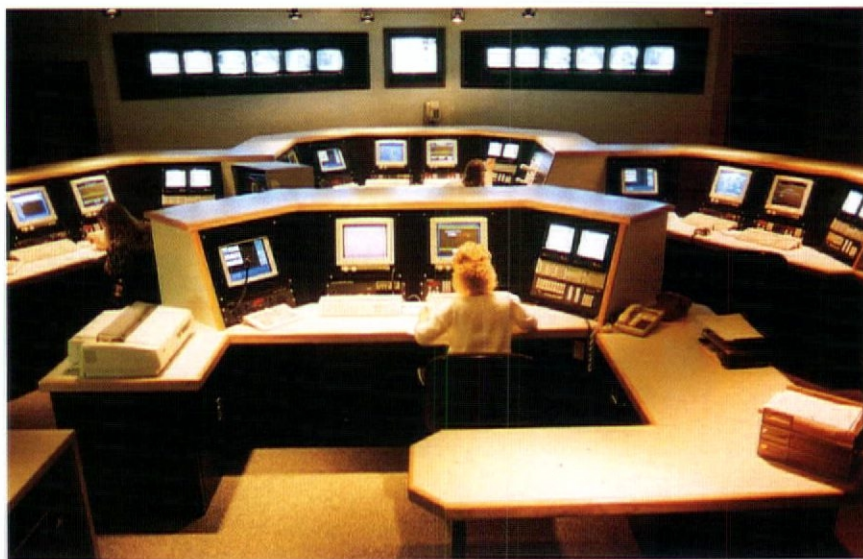
Space age security: Consoles such as this custom-designed model (above) by Mosler Inc., installed in the First Bank in Minneapolis, monitor access control systems and other security devices as well as security data input from 250 banking sites. The integrated system incorporates alarms with visual surveillance: A floor plan appears on the screen with a blinking light when an alarm is activated.
