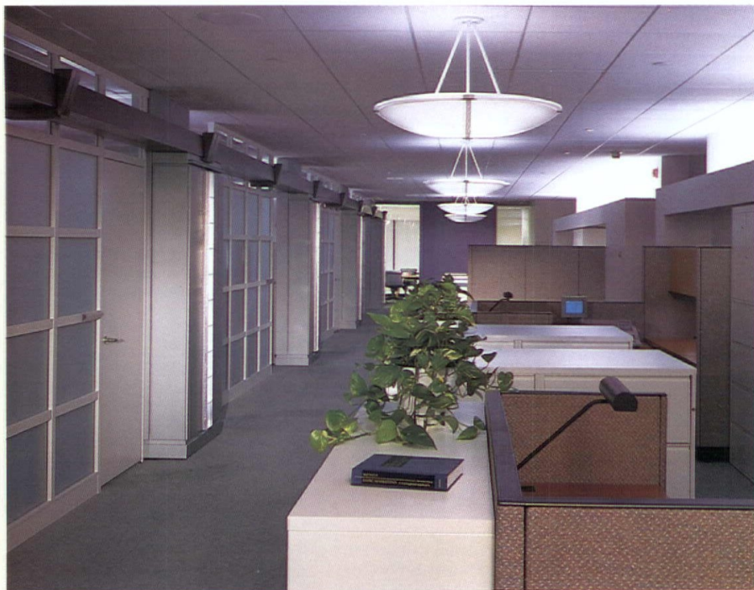
Running all around the main circulation corridor at Towers Perrin is an innovative, discreetly integrated open cable tray that can be seen at the transom level in this typical office floor view (left). Users of voice/data/power services can tap the tray for connections without disrupting office operations.
