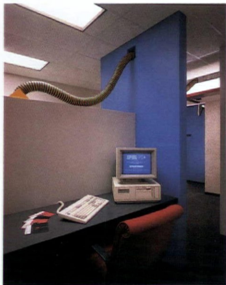
Mekus Johnson's whimsical application of color permeates this private work space (above), whether in furnishings, walls, cable tray trimmings, or the somewhat ominous cable hose suspended overhead.
