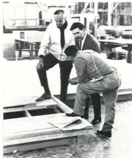
John Follis (l.), partner of Usher-Follis, and Dave Hammer, head of firm's design development, review showcase construction.
