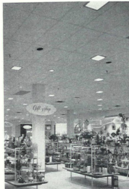
Figs. 9, 10. Massed or single-unit prismatic luminaires diffuse some light across ceilings to eliminate extreme contrasts and direct prescribed quantities of useful light to the occupant's viewing level. Desks and display items are comfortably illuminated, show form and texture.
