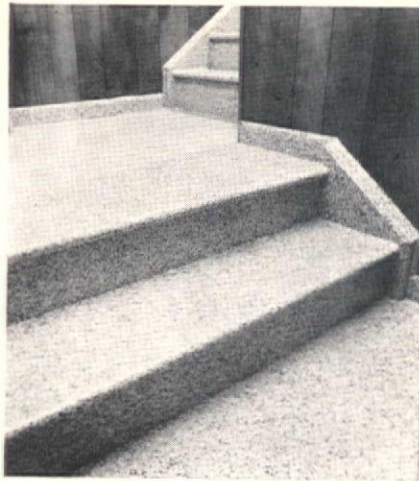
Seamless urethane was applied to a stairwell over wood and concrete including the stringers at sides. Installation was made in all hallways and stairwells of Hampden Medical Center in Conn.
