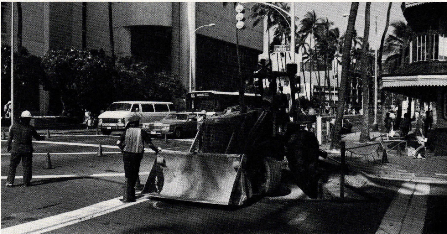
Construction of the project is now underway in Waikiki and should be completed in about 18 months. Photography by Rom Duran
