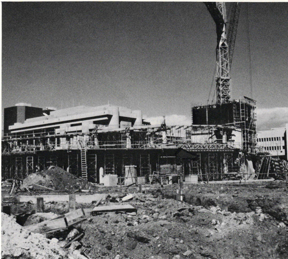
Construction on Bruce Stark's ONE WATERFRONT PLAZA in Kakaako is well underway.
