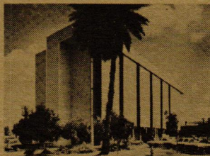
P H & M Building on Coral Street showing Montgomery hydraulic elevator exterior shaft installation on an existing structure.
