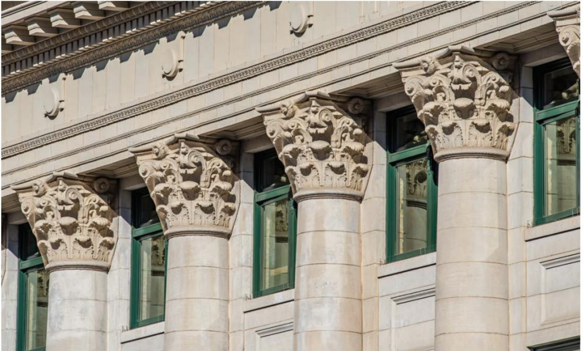
The Indiana limestone facade had suffered years of power-washing, sandblasting, and hailstorms that had pitted the surface and opened pores for dirt and water to penetrate. To address this wear, the stone's top layer was honed by hand to a smooth surface to resist dirt and water. Dishwashing soap removed the discoloration on other areas. / Photo: Tracy Allyn Photography
