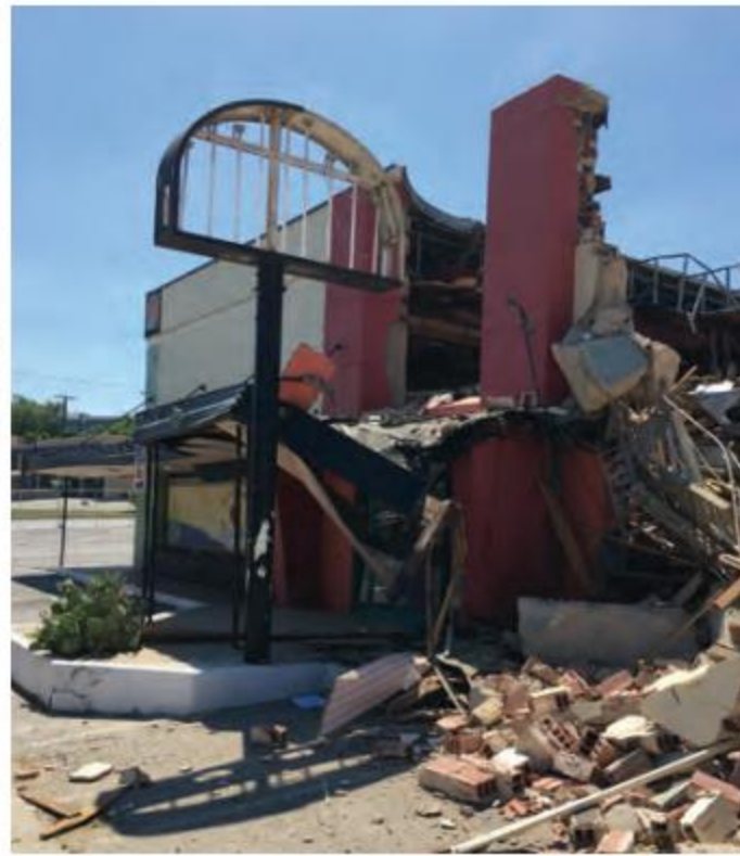
El Corazon, Oak Cliff: In the spring of 2017, the El Corazon de Tejas restaurant was demolished to make way for new development. Even though the building dated back to 1940 when it opened as a Wyatt's Grocery Store, there was little that could be done to prevent its loss. A demolition permit was pulled before the Landmark Commission could consider initiating the landmark designation process for the beloved Oak Cliff building. Photos: Preservation Dallas
