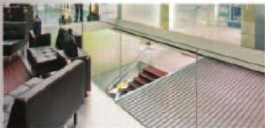
Horizontal Fire Shutters Zone-isolating fire shutters to prevent migration of heat/smoke/fire/toxins
