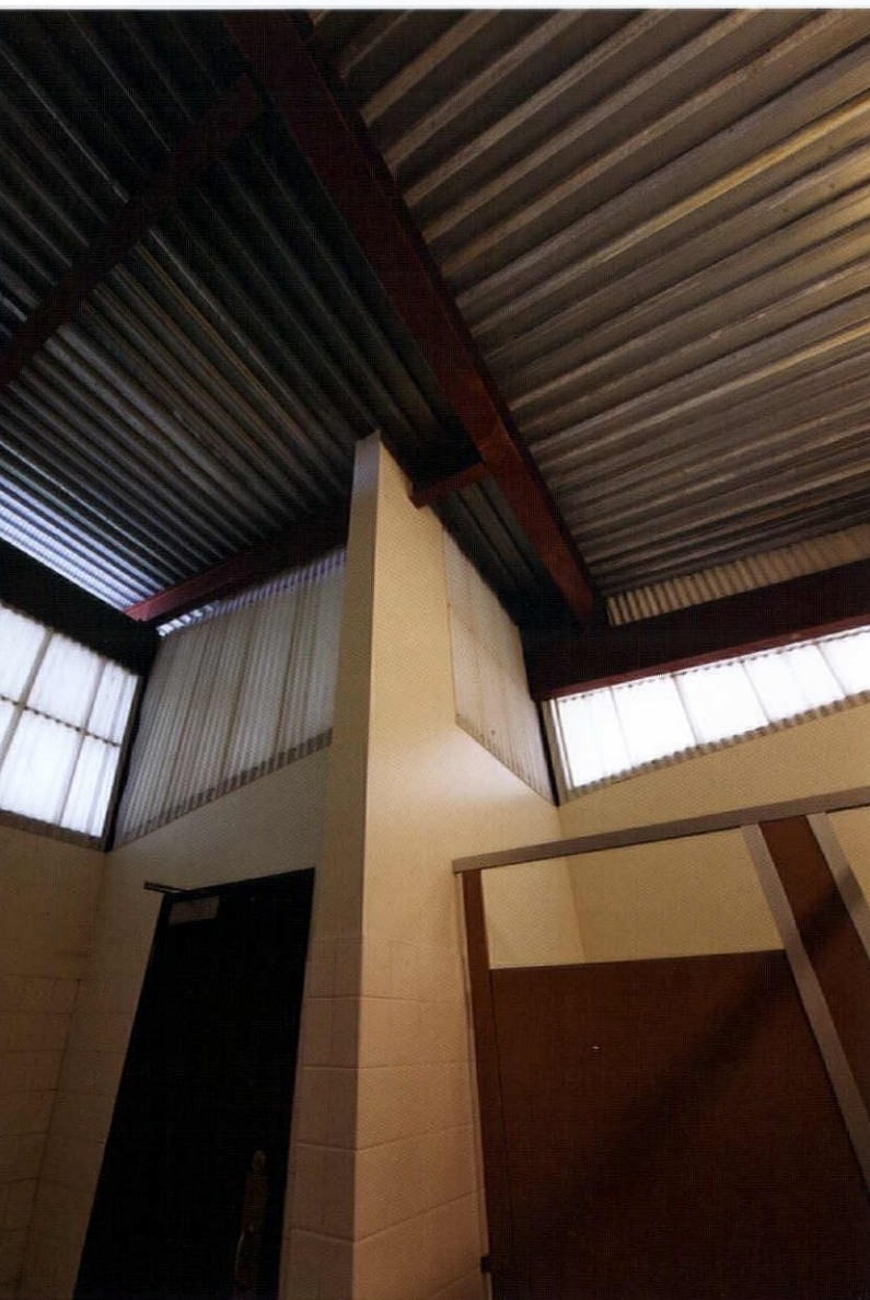
Below: Interior view from within the restroom facility towards the interlaced planes of steel decking and corrugated fiberglass panels at the roof level. The translucent panels help illuminate the restrooms and minimize the need for supplemental light.
