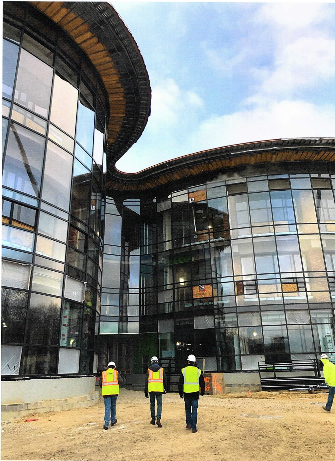
In fall 2019, SmithGroup participated in the Topping Off ceremony for the new R&D Facility for Promega Corporation in Fitchburg, Wisconsin. The project will be completed in fall 2020. SmithGroup is working in partnership with Uihlein/Wilson-Ramlow/Stein Architects .
