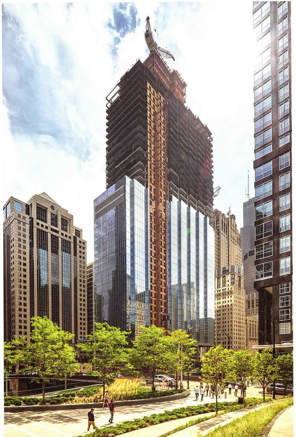
The Howard Hughes Corporation and Riverside Investment and Development hosted a celebration of 110 North Wacker's topping out. The 55-story office tower, designed by Goettsch Partners and built by Clark Construction , will open October 2020.
