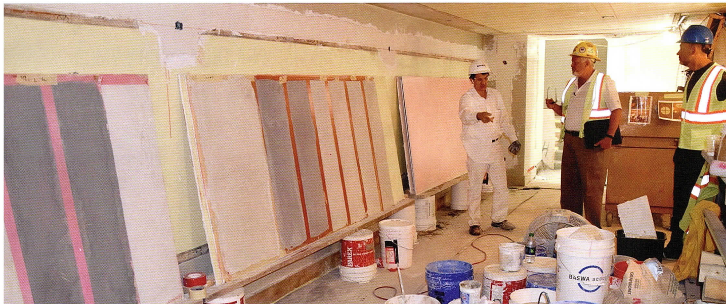
PLASTERER JOHN CZONKA OF J.P. PHILLIPS INC. AND MIKE HOOPER, PLASTERING DIRECTOR WITH INTERNATIONAL UNION OF BRICKLAYERS AND ALLIED CRAFTWORKERS DISTRICT COUNCIL #1 DISCUSS THE PLASTER SAMPLE PANELS.
