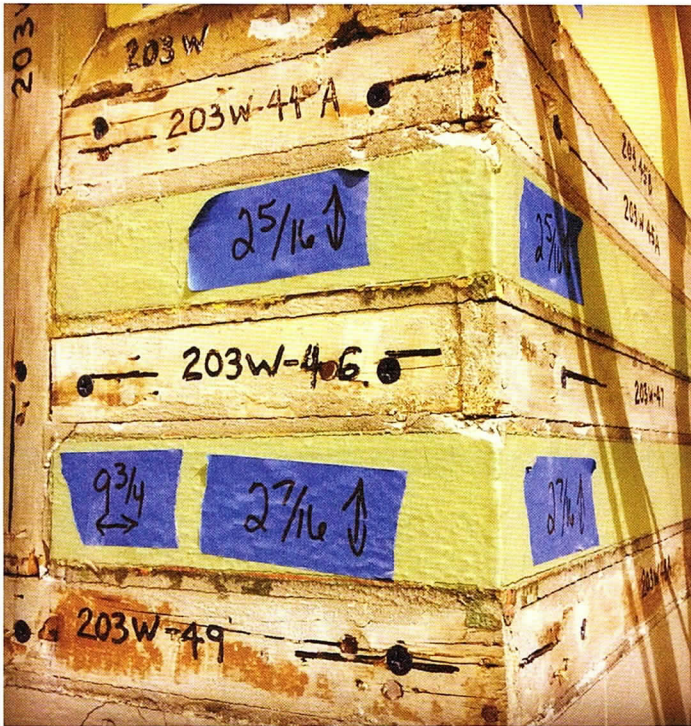
FORMERLY AFFIXED TO THE PLASTER, EACH PIECE OF WOOD TRIM INSIDE UNITY TEMPLE HAS BEEN PAINT-TAKINGLY REMOVED, TAGGED AND RESTORED OFF SITE TO BE REINSTALLED UPON COMPLETION OF THE PLASTER RESTORATION.
