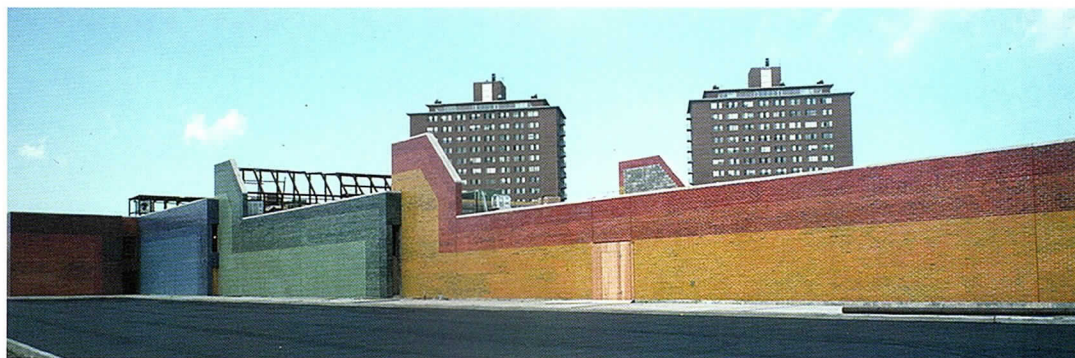
EXTERIOR VIEW OF THE NEWCITY YMCA WHILE STILL UNDER CONSTRUCTION, SHOWING THE MULTI-COLORED GLAZED BRICK FACADE AND PARKING LOT IN THE FOREGROUND. CREDIT: WILLIAM C. BRUBAKER, 1980. IMAGE COURTESY OF C. WILLIAM BRUBAKER COLLECTION (UNIVERSITY OF ILLINOIS AT CHICAGO) AT THE UNIVERSITY OF ILLINOIS AT CHICAGO. LIBRARY, SPECIAL COLLECTIONS DEPARTMENT
