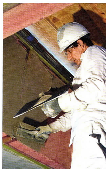
PLASTERER JOHN CZONKA APPLIES A FINISH COAT TO THIS CEILING COFFER IN UNITY TEMPLE.
