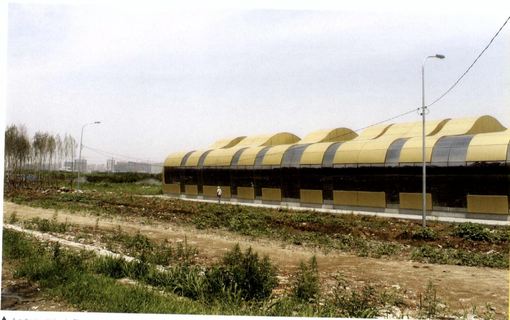
▲ A subway station in Shenyang, surrounded by unpaved roads. As officials plan for anticipated growth, China's emerging urbanism sometimes emphasizes quantity over quality. Although just three months old, the station had buckets situated throughout the lobby because of leaks.
