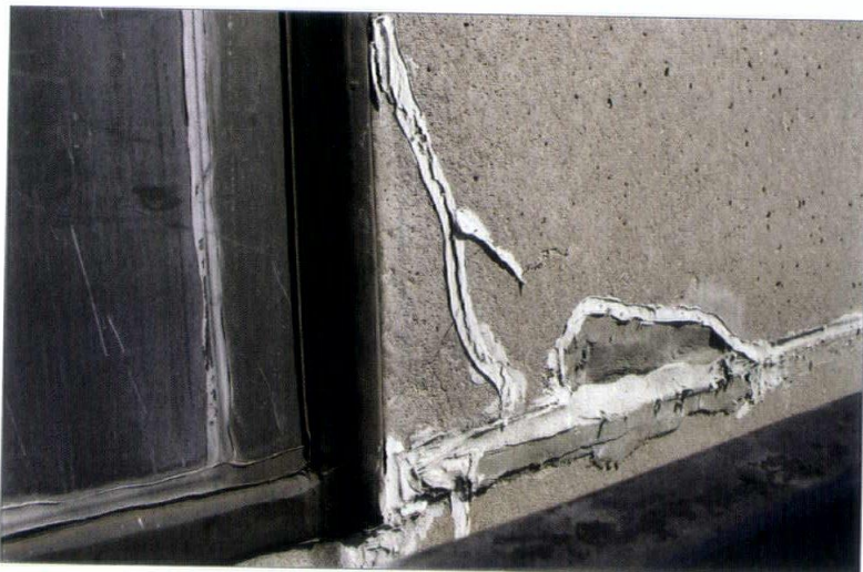
An inappropriate crack repair using surface-applied sealant. Many Modernist buildings used materials and construction techniques that are susceptible to long-term degradation due to corrosion, rot, mold and ultraviolet radiation.
