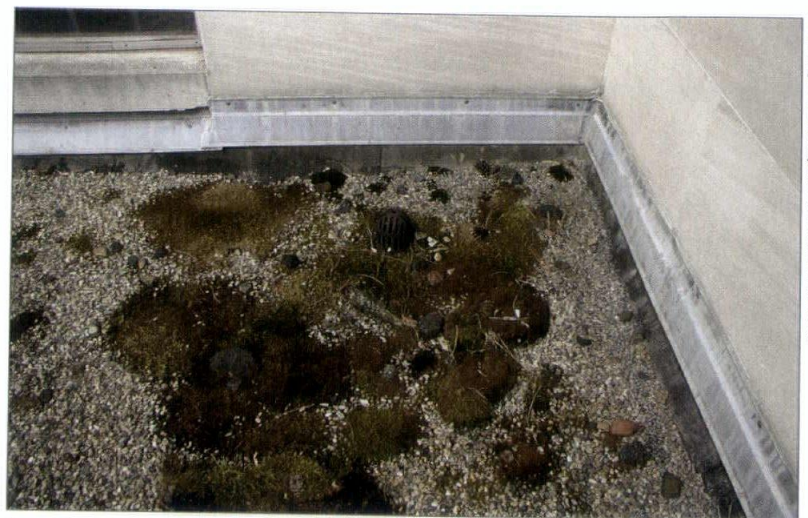
Organic growth and debris on the built-up roof of a Modernist structure. The materials and techniques of Modern architecture allowed for rapid and prolific construction, which resulted in a historically unprecedented volume of new structures during this period.
