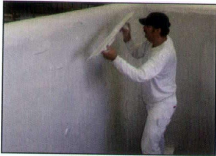
Conventional and Veneer Plaster
