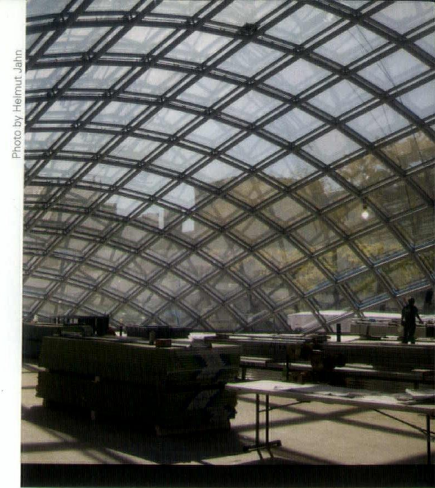
A view of the Mansueto Library during construction shows how the soaring, egg-shaped roof creates a lavishly daylight interior.
