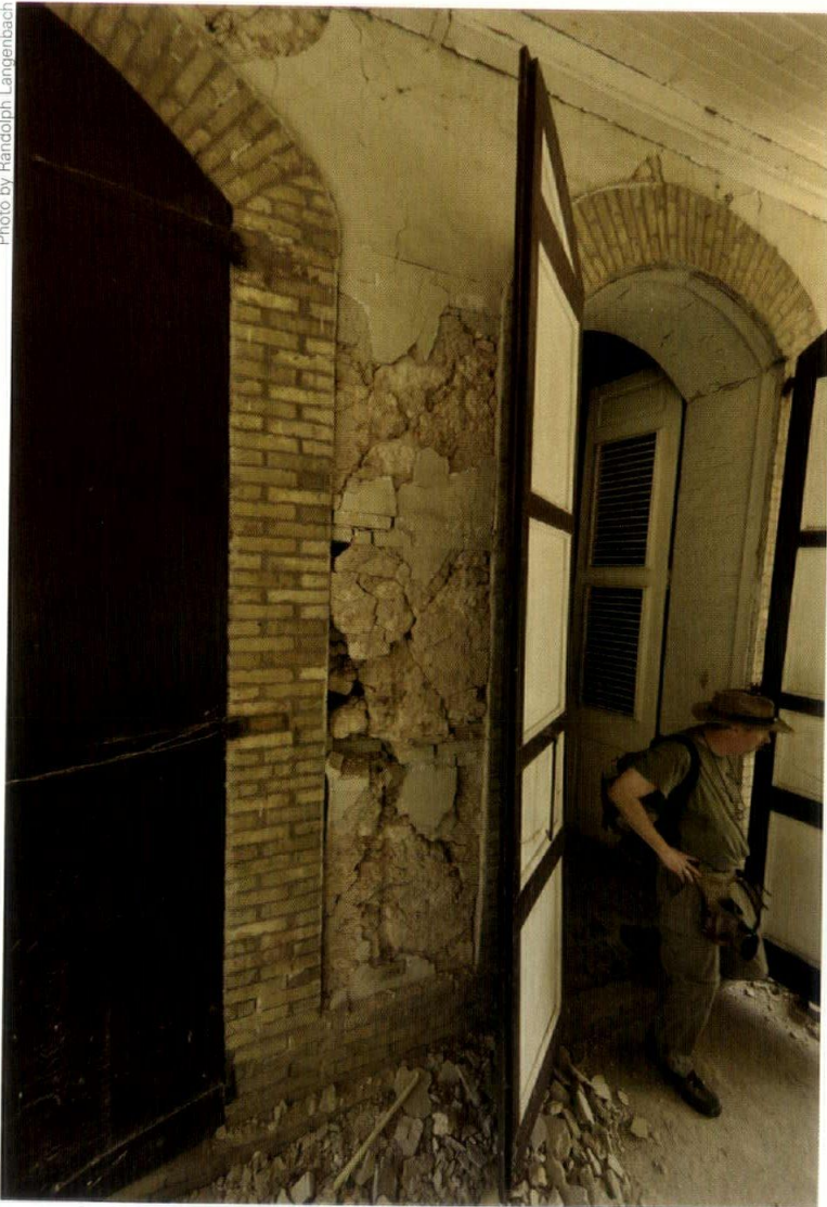
Stephen Kelley assesses a house. Each rapid assessment team inspected an average of eight structures each day.
