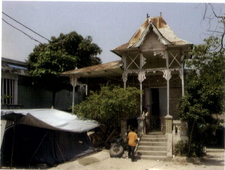
Kelley and his team observed residents who—afraid to live in their homes for fear the house might collapse—pitched and resided in tents on their property. After assessing this property, the assessment team declared the house safe for habitation.
