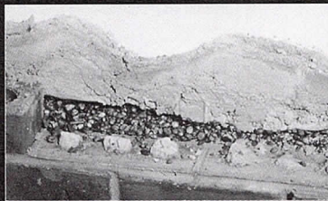
Damming and clogging of cavities can cause costly repairs due to water damage.
