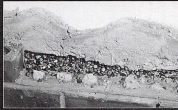
Damming and clogging of cavities can cause costly repairs due to water damage.
