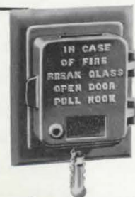
Fire Alarm Systems warn fire brigade of existence and location of fire.
