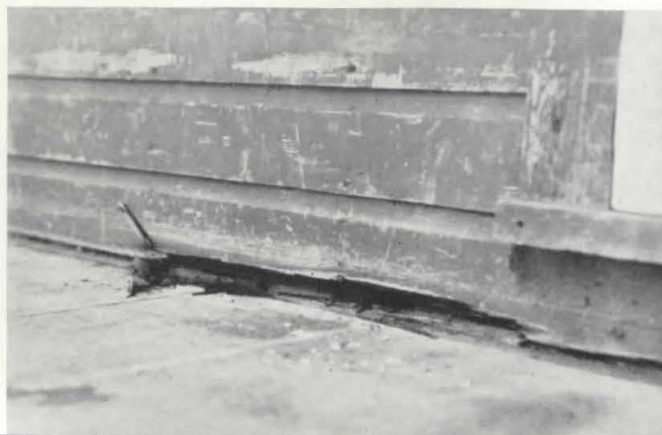
Right—expect this to happen whenever untreated wood is placed in contact with the ground, a concrete porch or sidewalk, or any other good source of moisture. Photo: courtesy of Forest Products Laboratory.
