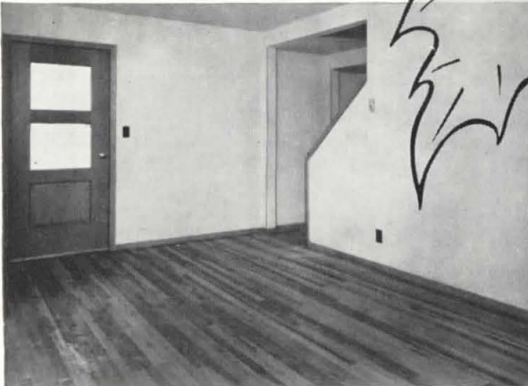
Southlawn Housing Project, Milwaukee. Architects: Ralph E. Schaefer, Frederick J. Schweitzer, George G. Schneider, Walter M. Trapp, Fritz von Grossmann. Contractor: Kroening Eng. Co., Milwaukee.
