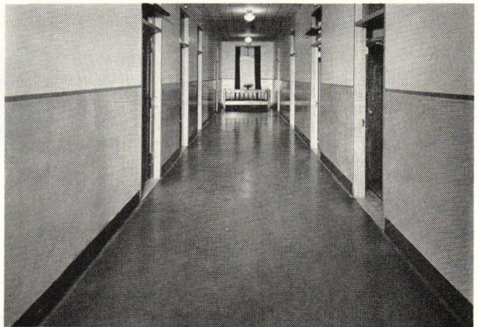
3. A corridor in the same hospital showing an installation of battleship linoleum now in use over thirty years! Proved long life where traffic is heavy . . . always clean and sanitary.
