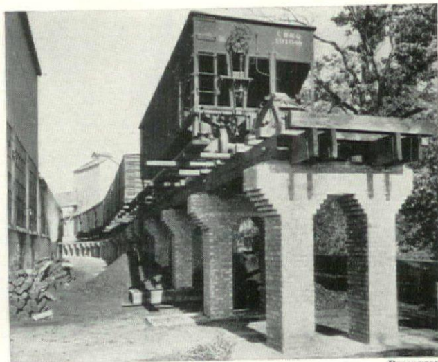
Reinforced trestle piers, built for the support of heavy loads practically without formwork.
