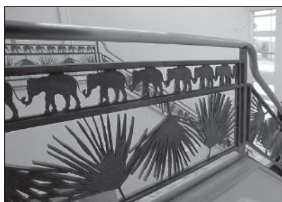
This elephant motif railing was created by Robinson Iron using water-jet-cutting technology.
