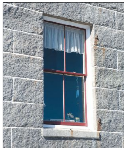
Architectural Components restored the double-hung windows to match the brick molding detail for the Customs House Maritime Museum in Newburyport, MA.
