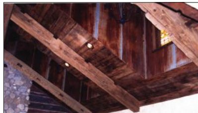
Hand-hewn beams and the antique roofers wood on the ceiling were both from Carlson's Barnwood ; the firm also supplied the antique stained glass window and the rusty antique corrugated tin in the dormers.
