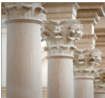
EverGreene created the historic plaster ornament for St. Thomas Aquinas church in Lincoln, Nebraska, including these capitals.
