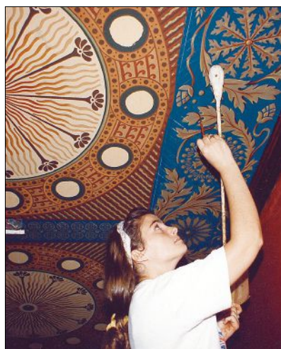
An artisan from Canning Studios works on the restoration of this decorative ceiling.
