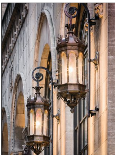
Allen Architectural Metals, Inc. restored the Exterior Cast Bronze Wall Lanterns of the Affinia Hotel in New York City.
