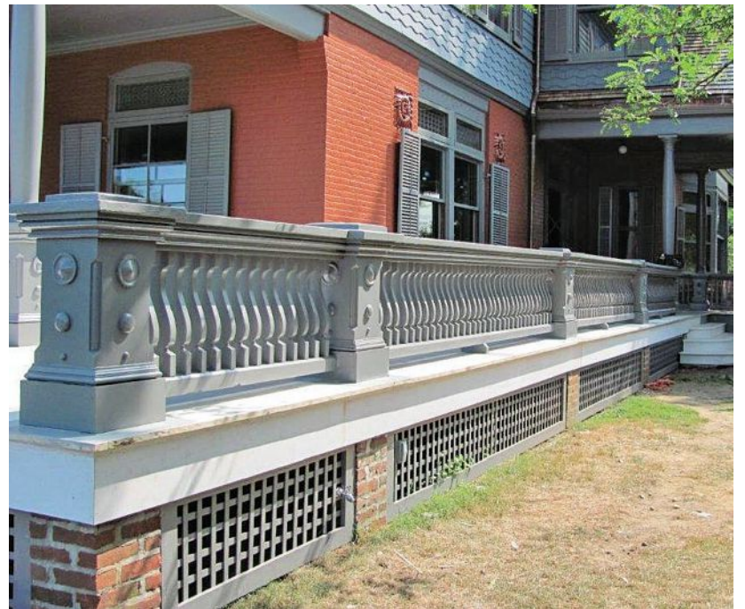
As part of a three-year, $7.2 rehabilitation, The National Park Service selected Accoya acetylated wood to replace the wrap-around porch at Sagamore Hill, Theodore Roosevelt's 1885 summer residence in Oyster Bay, N.Y.
