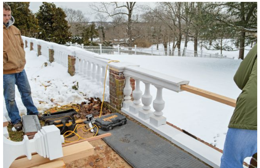
At Otlands Plantation in Leesburg, Va., the National Trust for Historic Preservation put acetylated wood to the test for reconstructing the balusters and cap of this weather-prone balustrade. PHOTO: Ashley Wilson.
