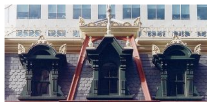
Custom finials from W.F. Norman were incorporated into the restoration design of this historic building in Toronto.
