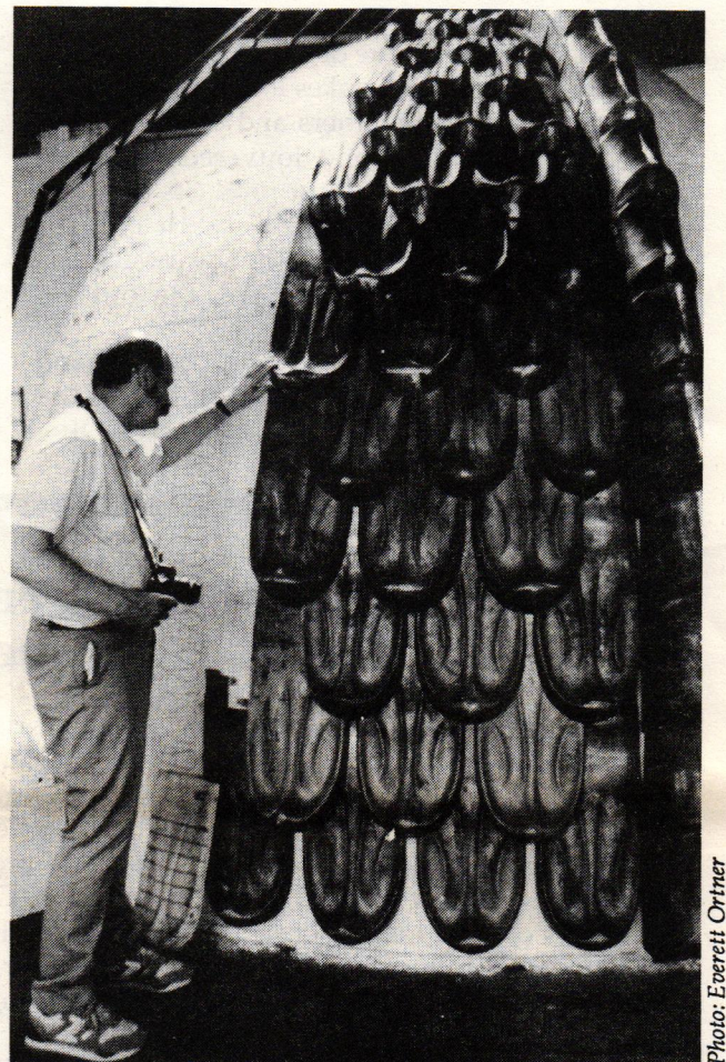
A 13-ft.-high full-scale quarter-section model of the Borough Hall dome was a vital tool in shaping each of the 14 rows of shingles, and in working out the system of copper clips to hold the shingles in place.
