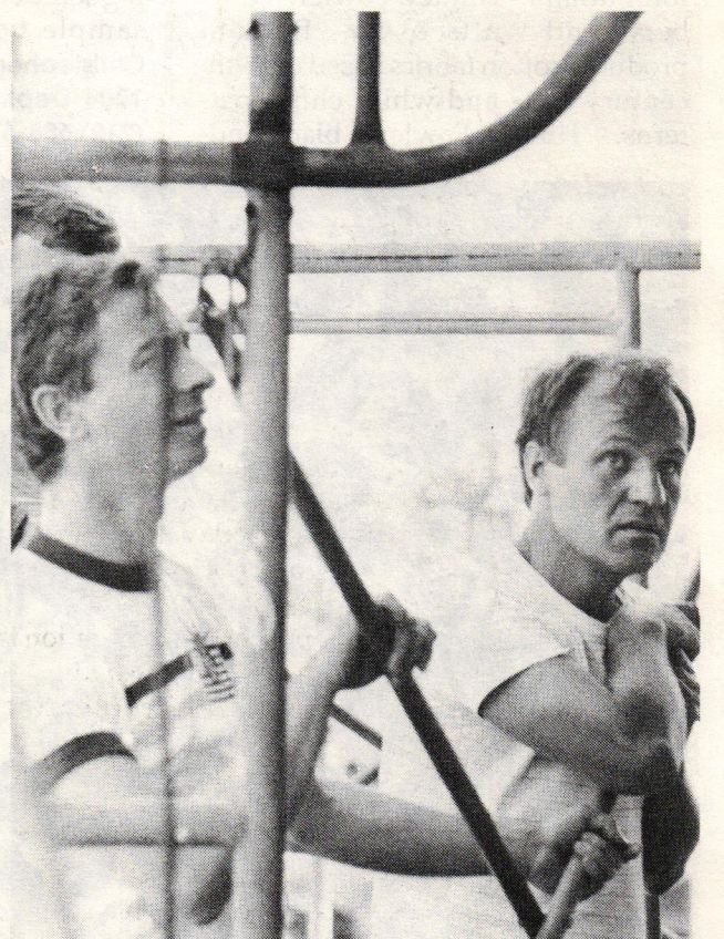
Jean Wiant, left, General Manager of LMC Corp., can frequently be found up on a scaffold providing close-up supervision of the metalwork installation process.
