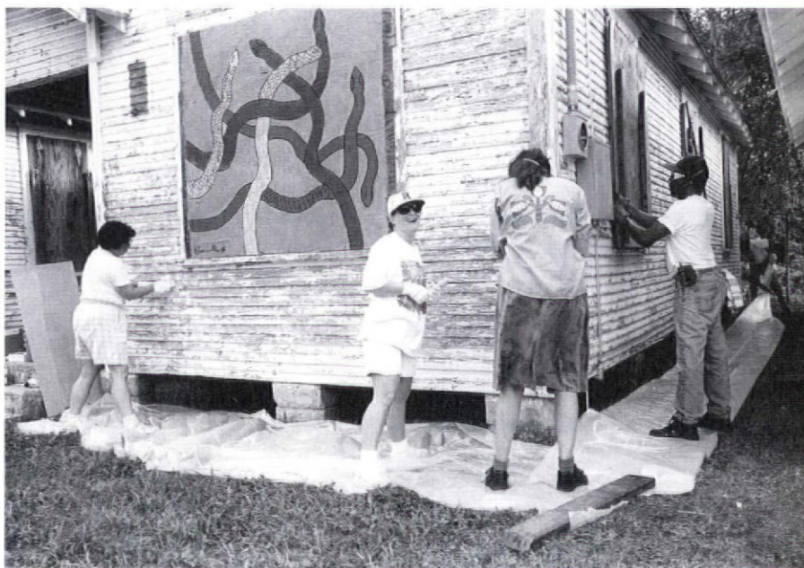
Volunteers refurbishing the exterior of the abandoned shotgun houses. (Stephen L. Clark)
