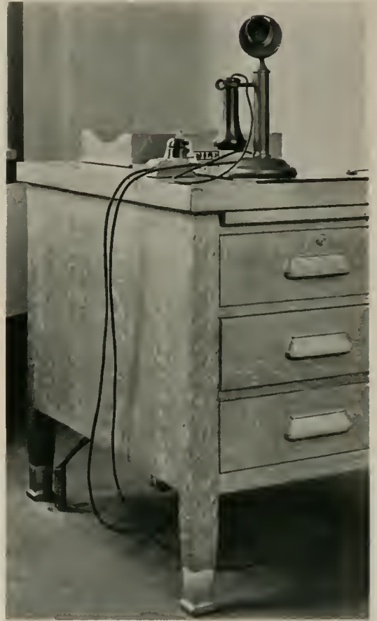
TYPICAL INSTALLATION, COAST DIVISION BLDG., P. T. & T. CO., SAN FRANCISCO
