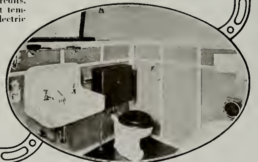
Bathroom in Residence of J. Horace McFarland Harrisburg, Pennsylvania Architect: T. H. Hamilton, Harrisburg, Pa. Contractor: John Myres, Harrisburg, Pa.
