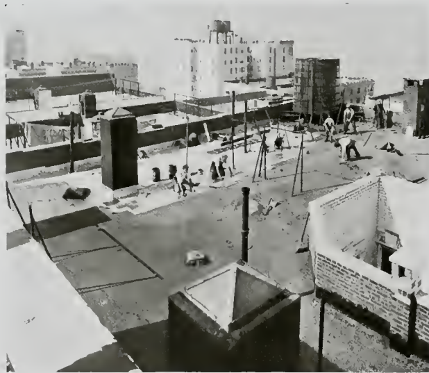
Roof of Trinity Terrace Court Apartment House, 152d Street and Broadway, New York City
