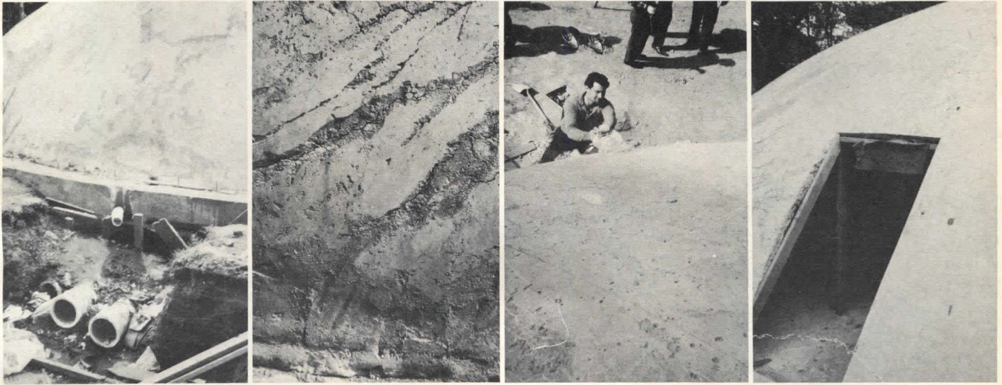
Left to right, above: Underground air lines, 8 in. in diameter, that inflated the elastic form. Shallow defects characterize exterior surface. Diamond saw cuts concrete and steel reinforcement. Rectangular access door that will be enlarged and formed into an arch.
