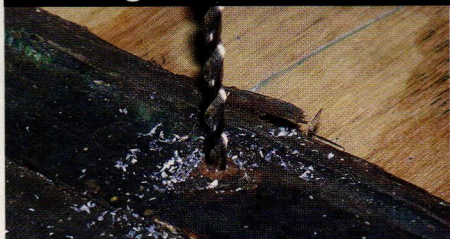
Remove old rivets by using successively larger drill bits to cut the existing peened end free.
