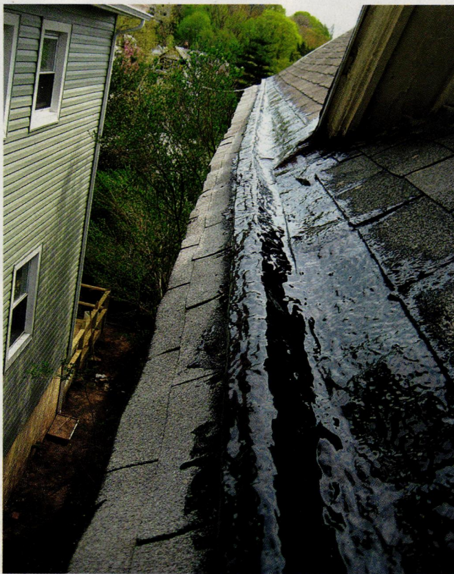
TOP: Use an ordinary paintbrush, a roller, or a squeegee to apply the activated rubber membrane along the length of the gutter, covering it completely with a thick coat. BOTTOM: The repaired gutter, with new protective membrane in place, will hold up for years to come.
