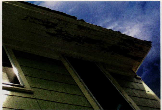
Damage from the problem areas was also visible from below, in the form of peeling paint and punky wood along the soffit.
