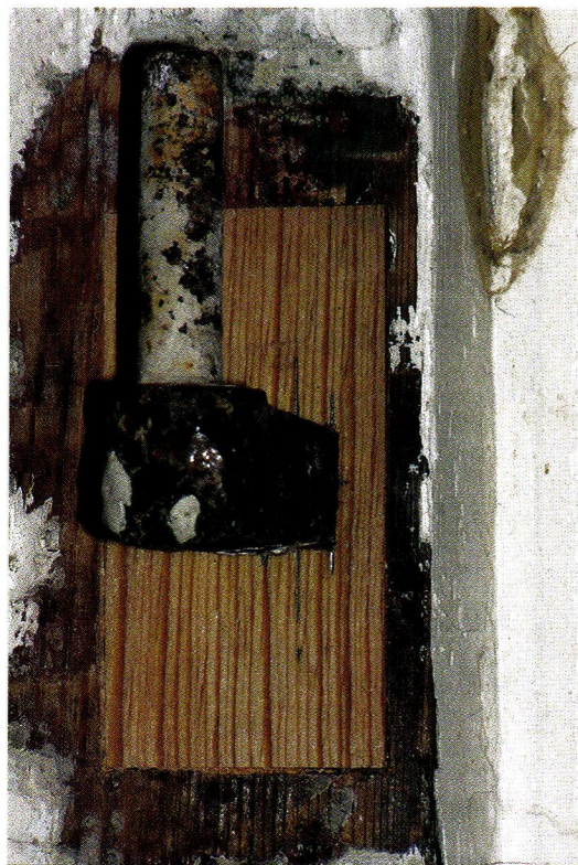
After verifying that the tang fits securely in the new mortise, you can paint the jamb to create a virtually seamless repair.
