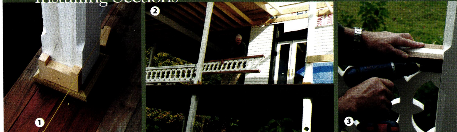
Now ready to install an entire section of railing, Jim first used a string line to ensure that his support blocks were in square (1), then he carried the railing section into position and slid it into the grooves on the support blocks (2).
