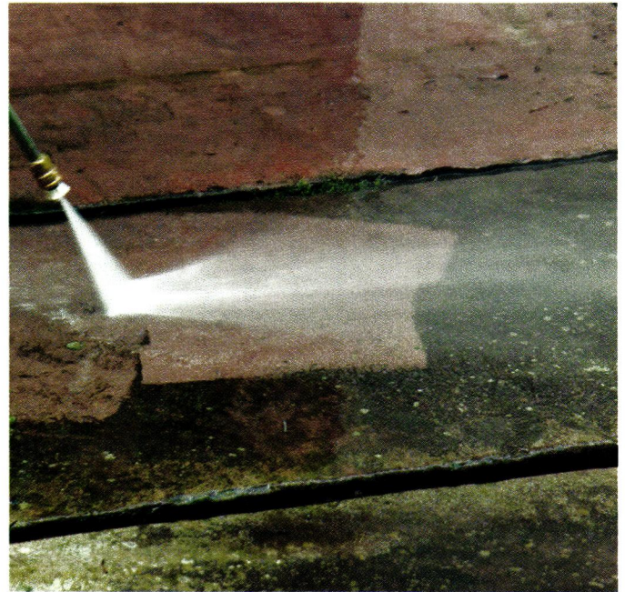
To clean away years of grime and better evaluate the condition of the original Medina stone, the team used a pressure washer to thoroughly scrub its surface and uncover the original reddish-brown hue.
