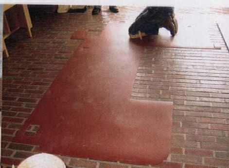
Before installation, Norris meticulously trimmed the linoleum to size, making cutouts where the counter intersects electrical outlets.
