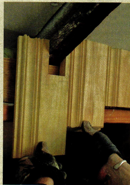
The finished piece fits snugly around the rafter. Mapping out the notch on a scrap first, then copying it on the finished piece, ensures a perfect fit.
