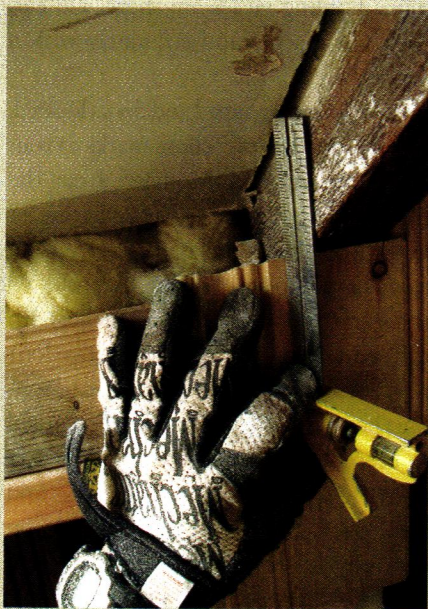
Fitting the tongue-and-groove paneling around the rafters requires making angled cuts in three planes. Start by transferring rafter measurements to panel stock using a 7" bevel square.
