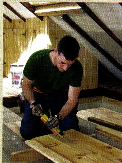
Square a line, dab some construction adhesive, and place the 1x4 rail (rails should be 2" shorter than door width) on the line.
