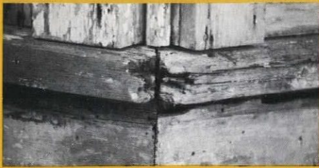
This rotted – and irreplaceable – woodwork...
