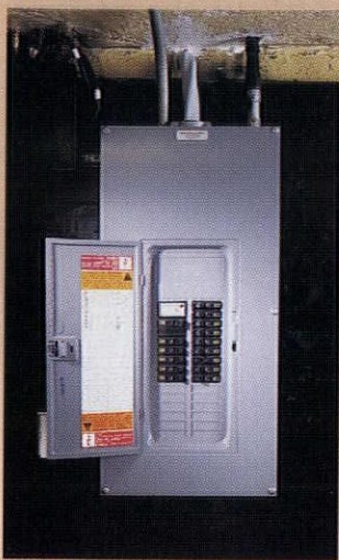
This modern service panel, with all breakers in a single enclosure and labels on the inside door, is easy to understand in an emergency.
