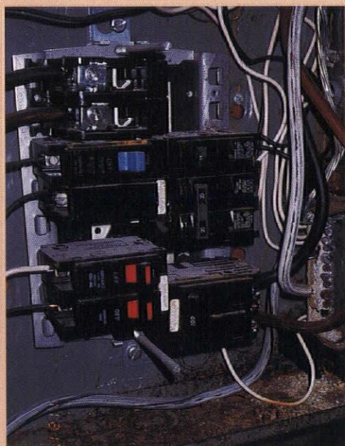
Excessive rust such as this may indicate that rain is entering the panel box. Weatherproof all outdoor penetrations with duct seal putty and exterior-grade sealant.
