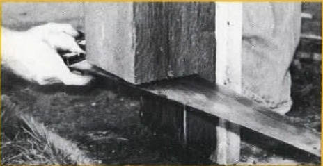
10" rotted bottoms of these load-bearing columns...
