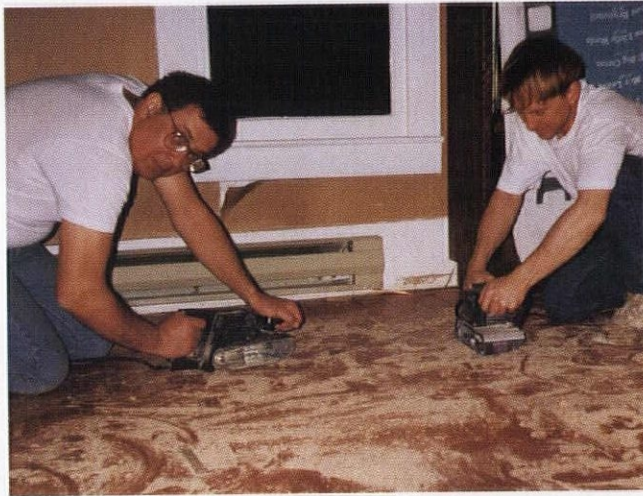
Here, Dave and Jim pose with part of our sander arsenal. At the time, we rarely stopped working because a break meant risking a chill in the cold room.
