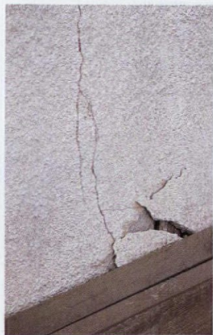
A vertical crack indicates a structural problem underneath. In this case, the foundation had given out.
