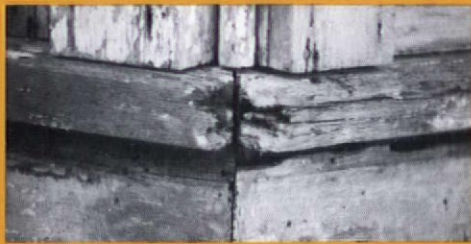
This rotted – and irreplaceable – woodwork...
