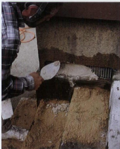
Lay sand on surfaces underneath your work area to prevent spilled mortar from sticking. You want the first coat to ooze through the lath for a good grip.
