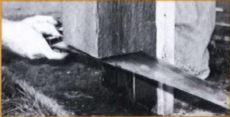
10" rotted bottoms of these load-bearing columns...
