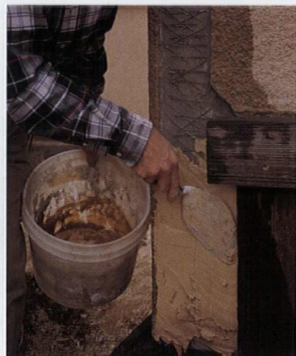
The final coat should be a thinner mix so it can take the texture. Get a solid coat on the patch and let it harden slightly before texturing.
