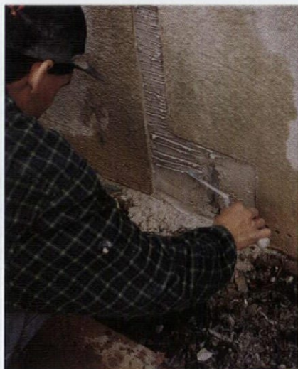
The second coat should be only slightly below the plane of the wall. Key all undercoats to give upper layers something to hold.
