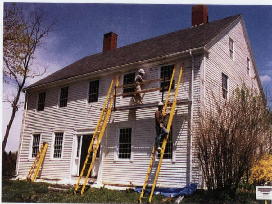
Regular paint maintenance, like spot scraping and painting, has kept this house in good condition for more than 200 years.
