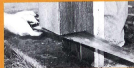
10" rotted bottoms of these load-bearing columns...
