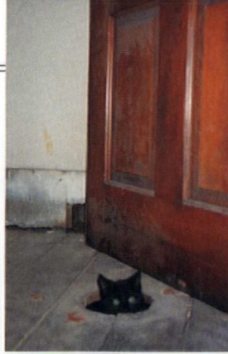
Reader Joan Lee's cat Alice disappears into a plumbing hole — once a toilet, oddly situated in the middle of a hallway.
