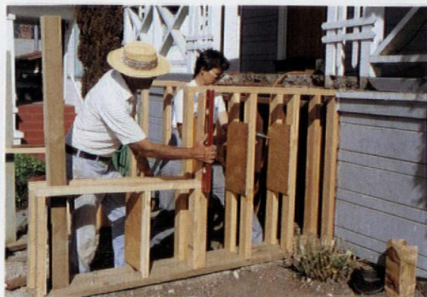
Each wall was two 2x4 frames tied together with plywood. Sills were treated lumber anchored to the old masonry footings.
