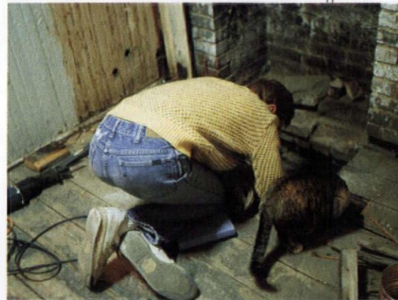
Alan Doyle and Io peer into the basement, trying to figure out how to support a new section of floor.
