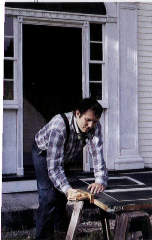
Final trimming on the bottom of the door to fit the new sill.
