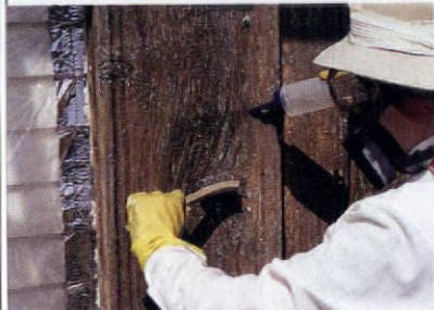
An alcohol rinse removes the last residue of chemical remover while masking protects the adjacent surface.
