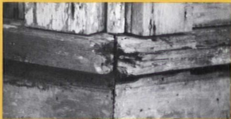
This rotted – and irreplaceable – woodwork...
