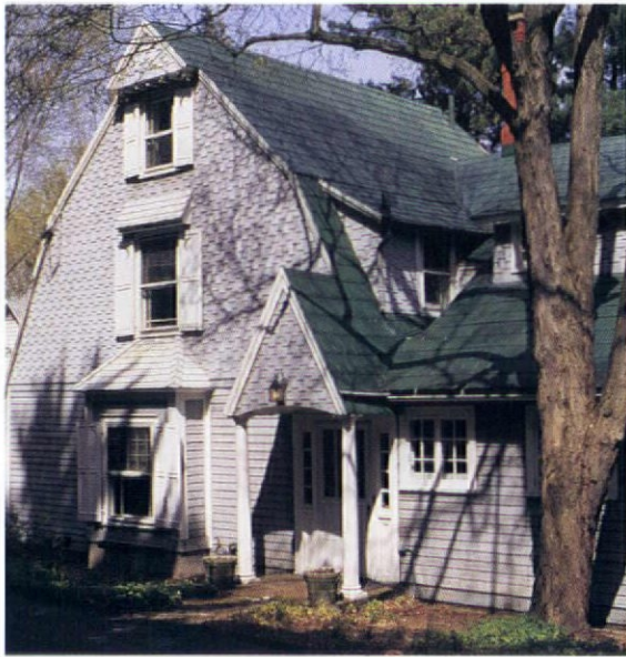
This c. 1900 Shingle-influenced house in Nyack, N.Y. still sports its original roof of "Queen Anne" metal-shingles.
