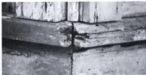
This rotted – and irreplaceable – woodwork...
