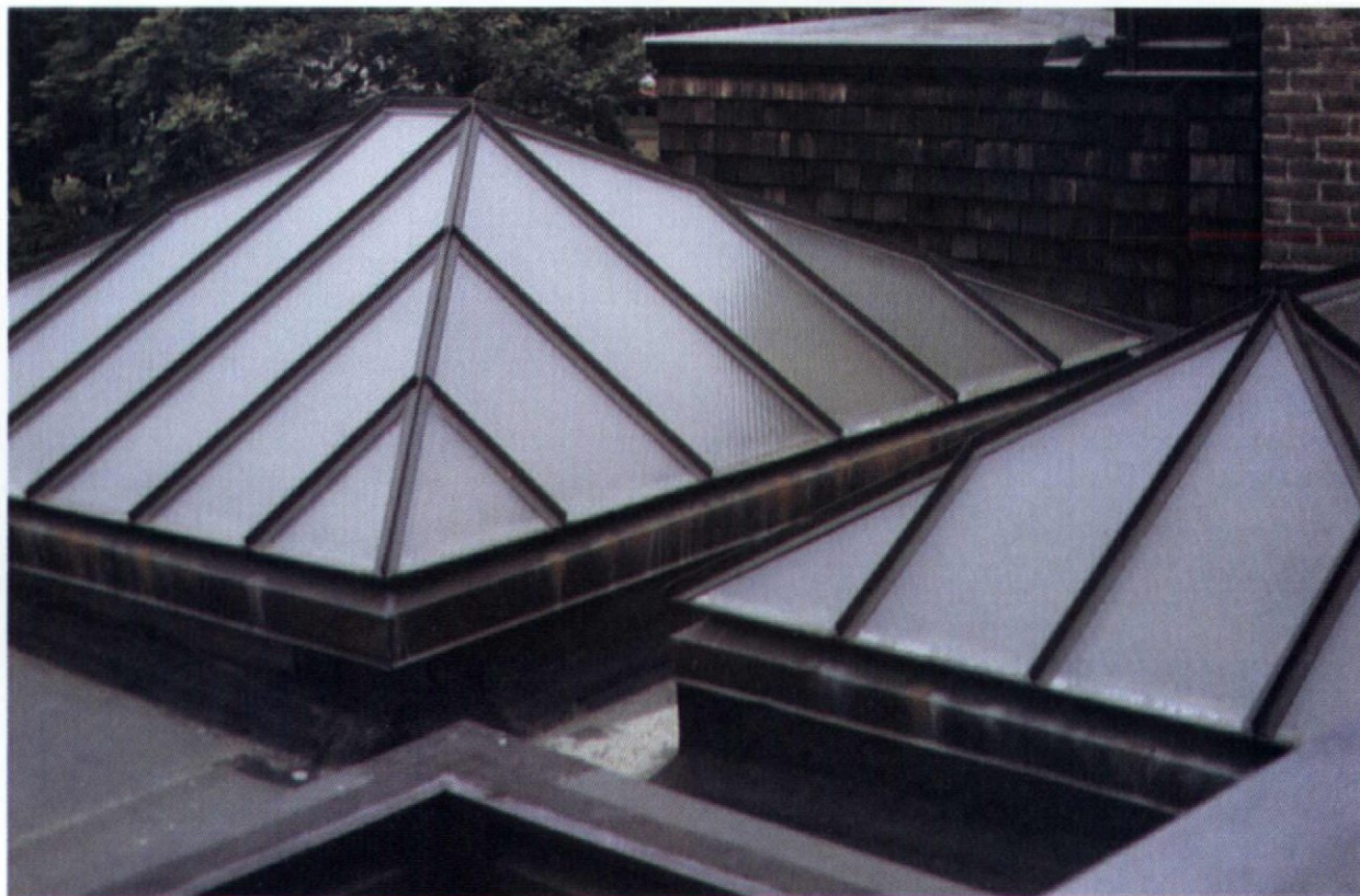
Restored skylights at the Frank Lloyd Wright home and studio in Oak Park, Illinois.
