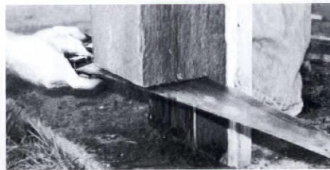
10" rotted bottoms of these load-bearing columns...
