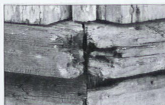
This rotted - and irreplaceable - woodwork...
