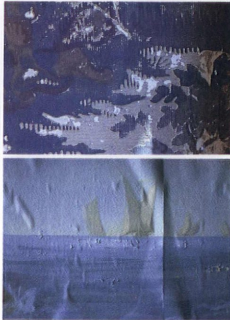
Two examples of wallpaper problems most homeowners cannot address: insect damage (top) and bubbles of detachment (above).
