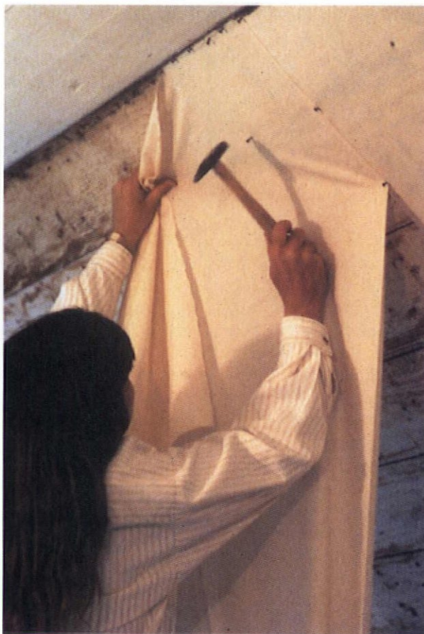
When netting a room, position tacks as needed to keep the fabric smooth, avoiding cracks between boards. Plan fabric runs so there are no horizontal seams (which can buckle or fail).
