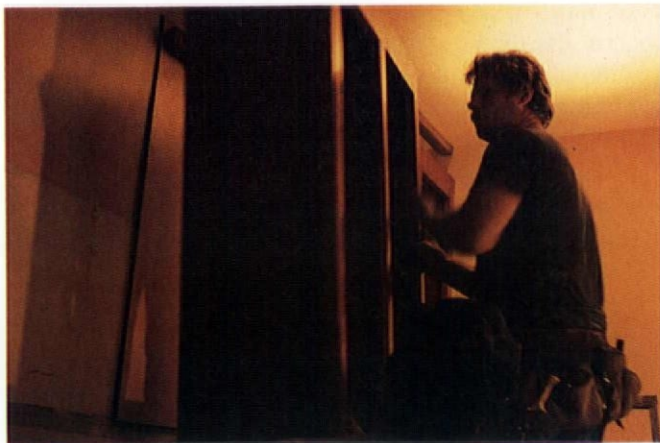
Lifting a cabinet onto its clinch bar and back.
