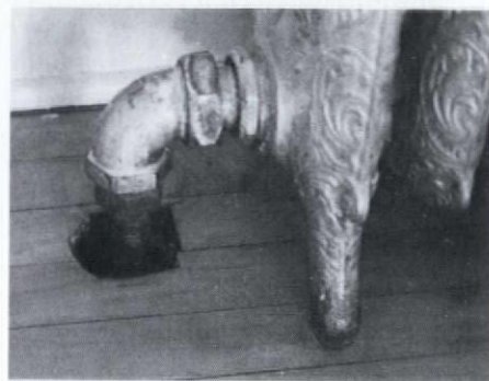
A split-ring escutcheon is needed here.
