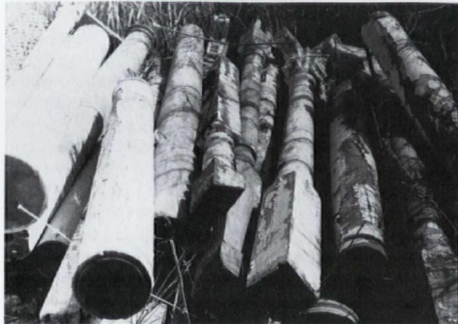
Salvaged columns are easily inspected for rot at tops and bottoms when laying on the ground.
